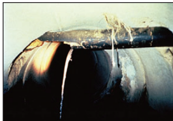
Figure 1: Sewer Pipe Discharging to the Storm Drain System
